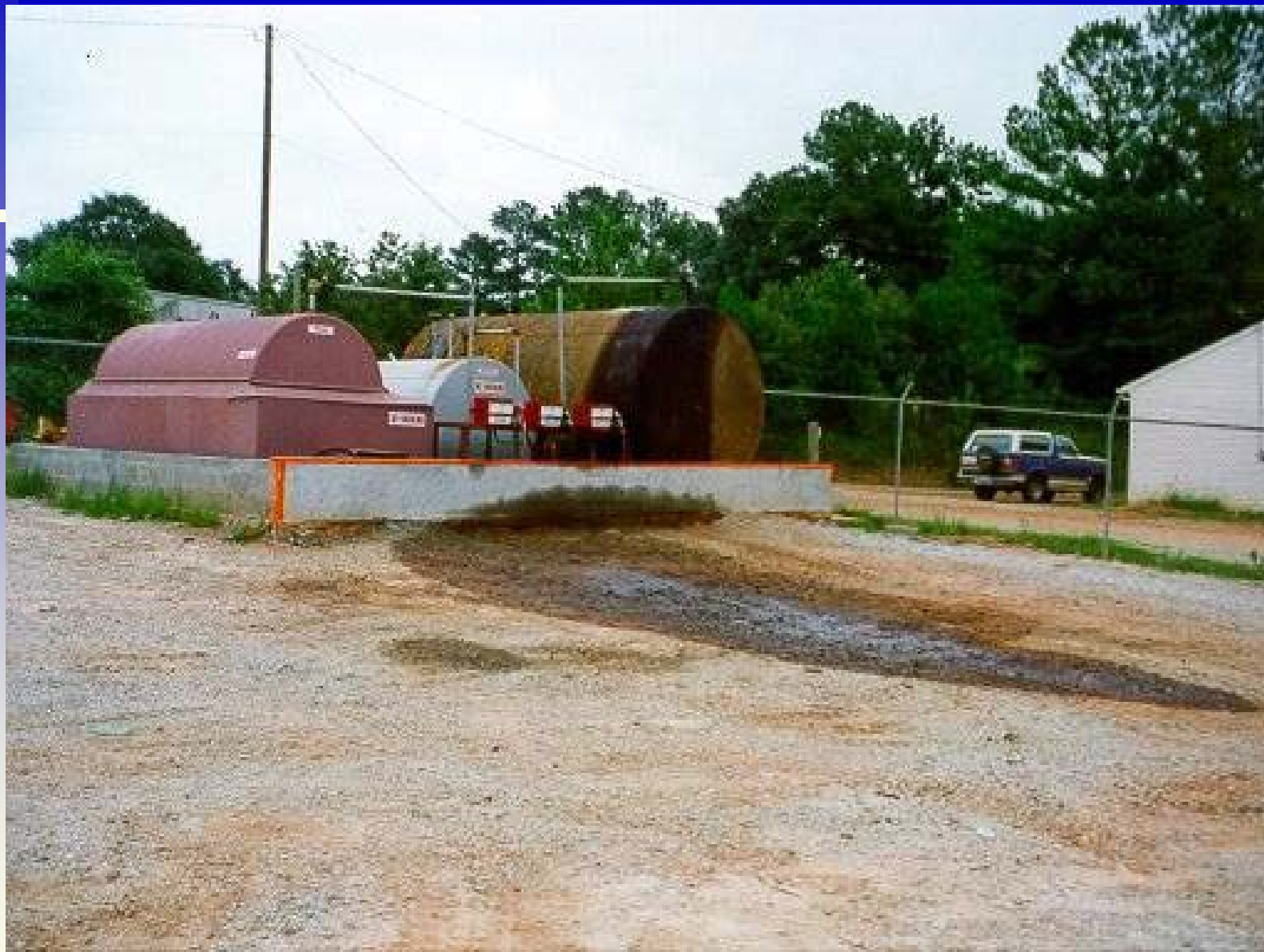
Inadequate Containment and Overfill Protection
